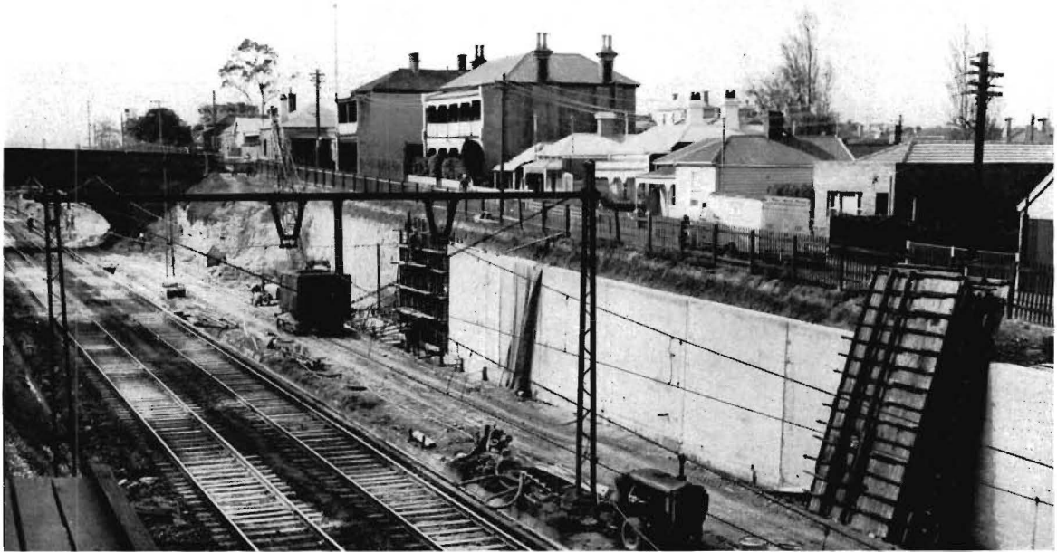
Construction of retaining wall to provide for additional tracks between East Richmond and Burnley
